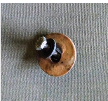
Fig 14 – One of the window frame lower mounting bolts and the factory spacer.
